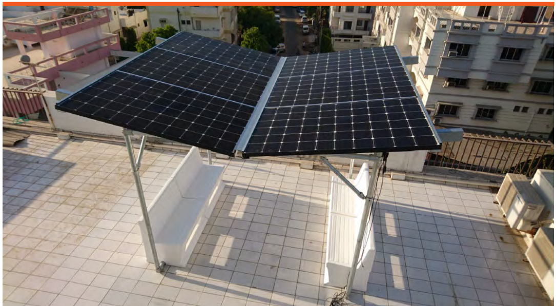
PV Port System installed in Gujarat.
