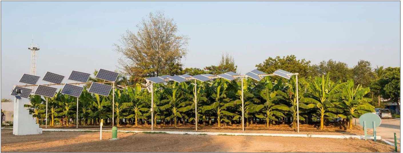
Figure 13: 14.4kW agrivoltaic structure with banana (Credit: Jain Irrigation)
