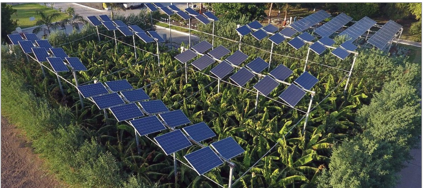
Figure 14: Aerial view of 14.4kW agrivoltaic structure with banana (Credit: Jain Irrigation)
