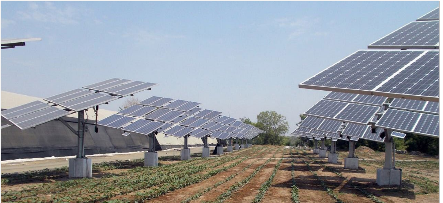
Figure 15: Agrivoltaics with tracking and drip irrigation (Credit: Jain Irrigation)
