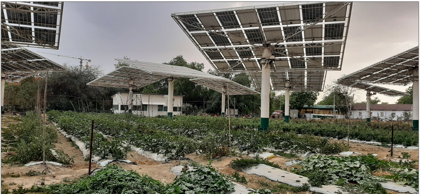
Figure 6: Dayalbagh Agriculture University agrivoltaic plant (Credit: DAU)
