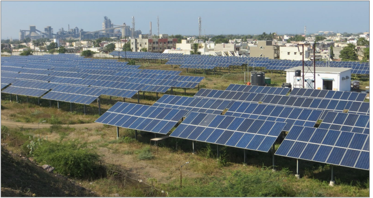
Figure 6: Harsha Abakus 1 MW Sikka plant (Credit: NSEFI)
