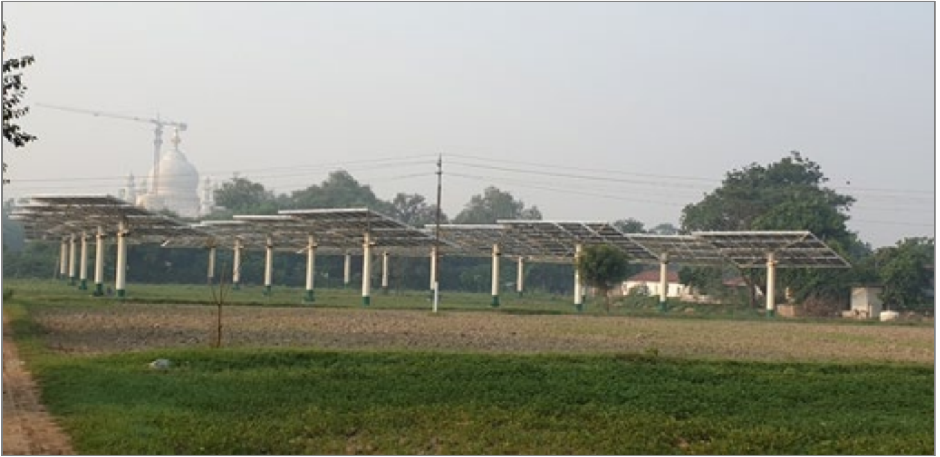
Figure 5: Dayalbagh Agriculture University agrivoltaic plant (Credit: DAU)
