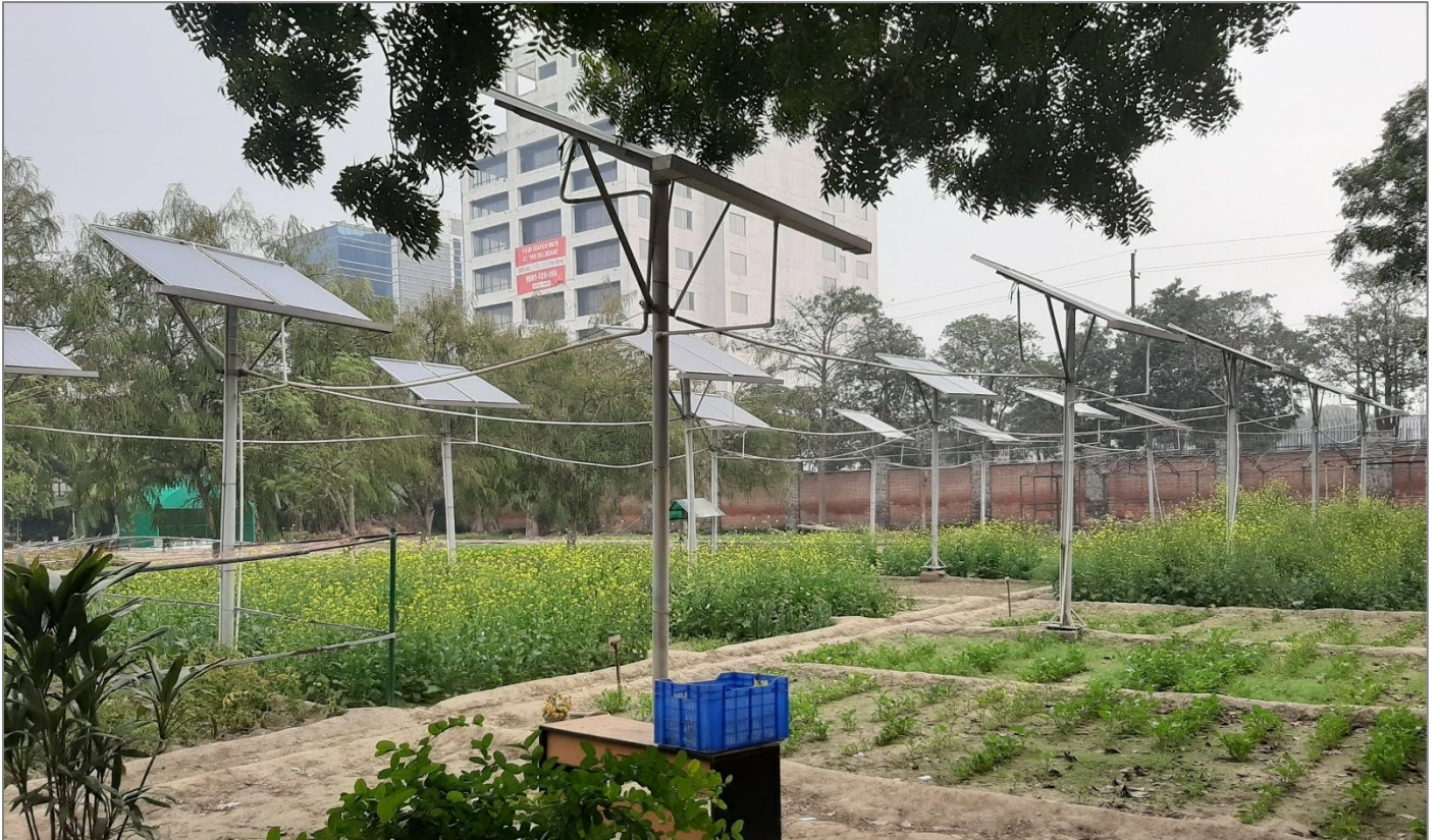
Figure 4: Plant at Amity University (Credit: NSEFI)
