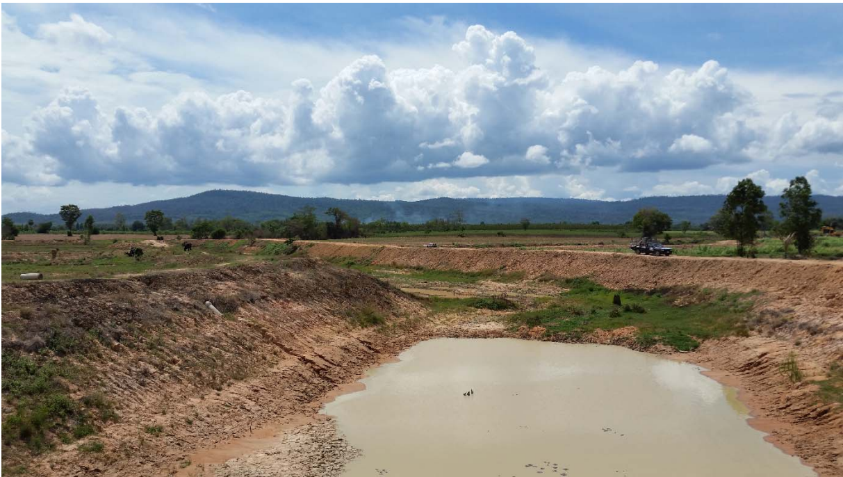
Figure 29: Dikes along the embankment, embankment with bare soils
