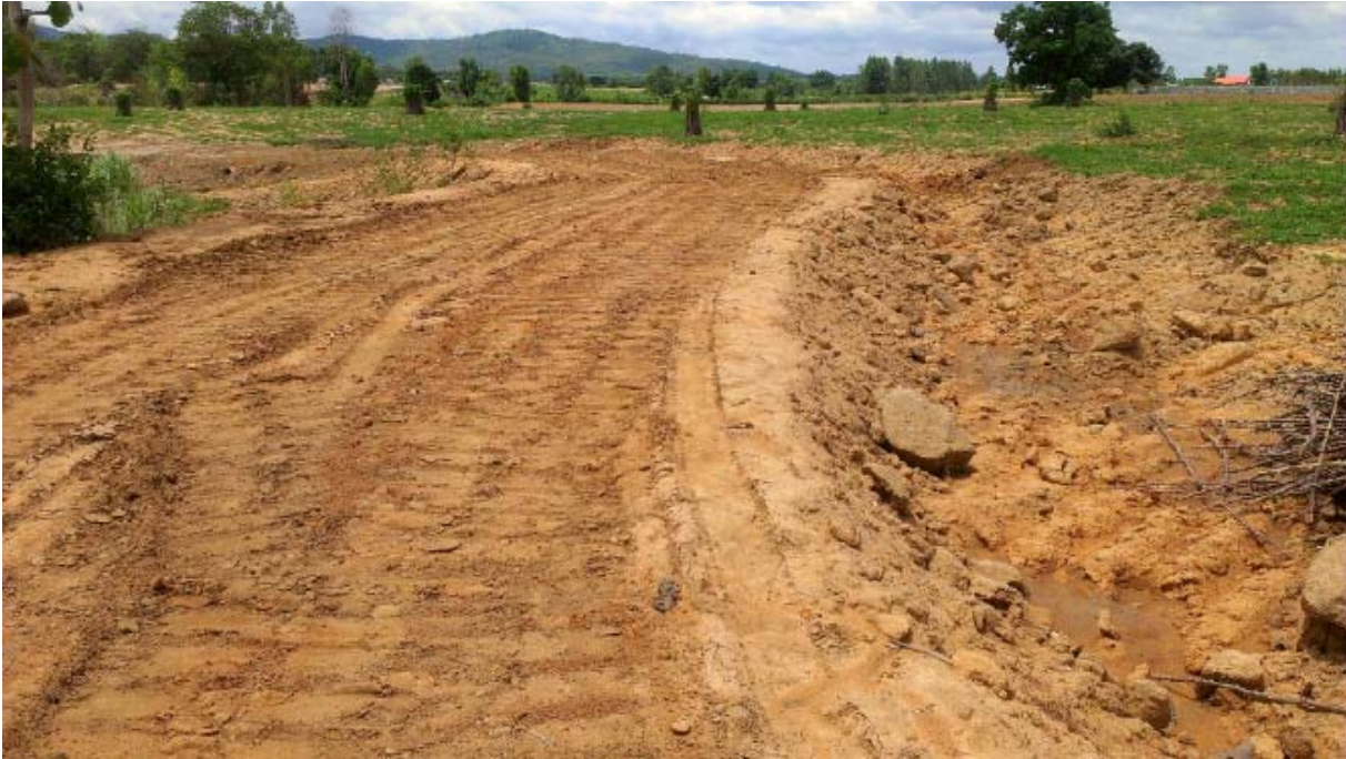
Figure 25: Erosion from road with the farmland area
