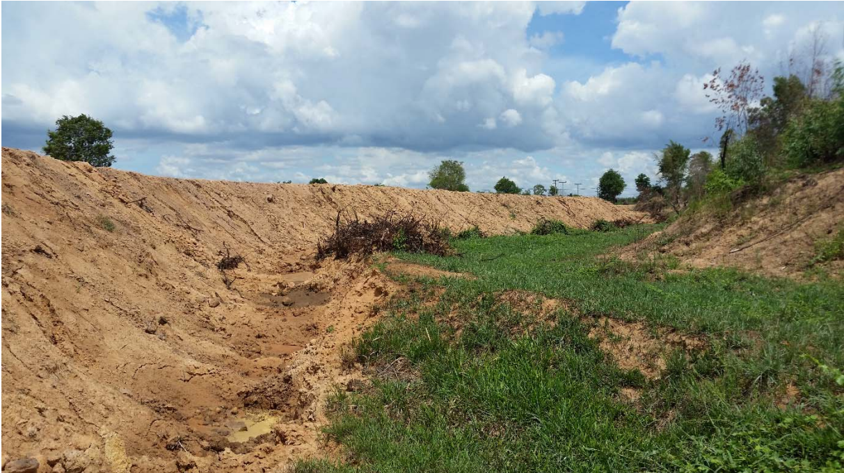
Figure 30: Erosion of river embankments
