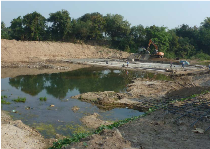
Figure 6-10. Construction of a concrete weir in the Lam Pa Chi river. Author: Santiago Penedo
