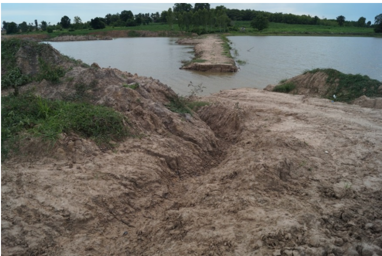
Figure 5-7: Severe erosion of sediments dredged from the reservoir and dumped in the immediate surrounding of the Nong Yai reservoir (Photo: T. Zumbroich, 2015).
