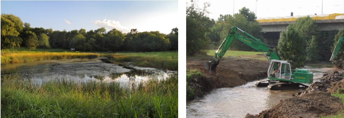
Figure 5-10: Example of a fully developed sediment pond (left) (Source: http://saveourstream.blogspot.de/p/sediment-ponds.html ) and construction works (profiling and widening cross-section profile) for the installation of a sediment pond (right) (Source: Zumbroich Consulting)
