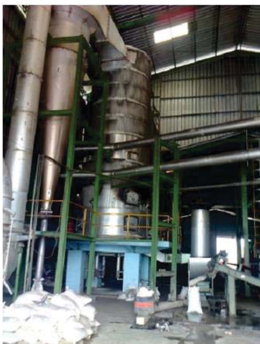
Coal-powered drying unit at the tapioca starch plant of PT. SPM
