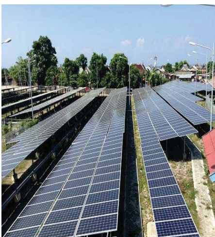
The solar PV plant at Kodingraeng island
