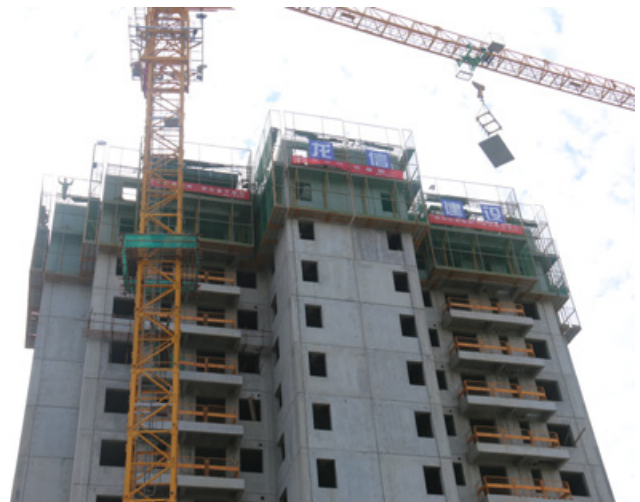
Installation of prefabricated concrete components for the Nantong Longxin Square project in Jiangsu Province, China 中国南通市龙信广场项目预制混凝土部件安装现场 Source / 图片来源: CSTC
