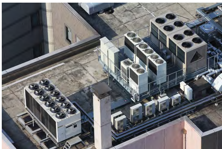
Green Chillers introduces green cooling technologies to industry and residential areas. The picture shows cooling systems used in residential areas. ©GIZ
