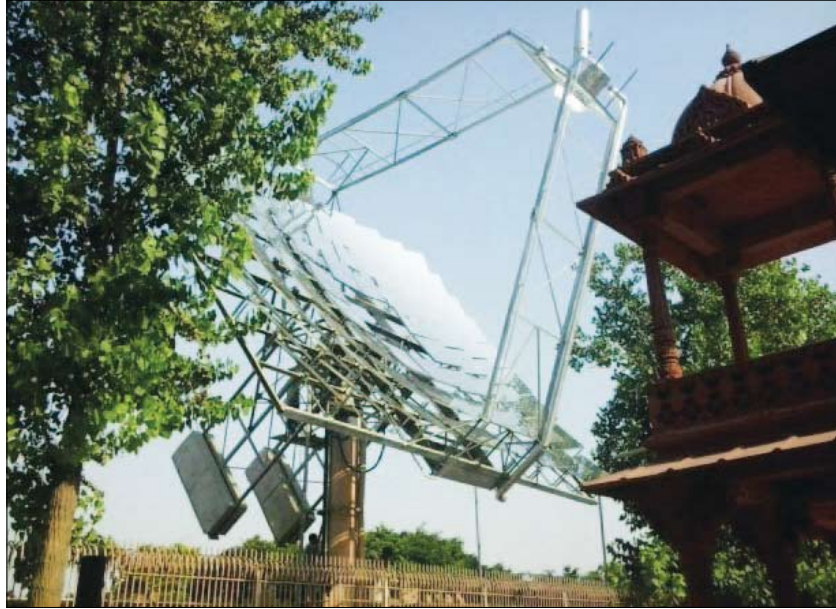
Image no. 3-22: Example of renewable energy application for steam generation at Akshar Dham temple, New Delhi for community cooking 46
