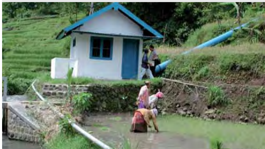
This picture shows the turbine house of a micro hydro power facility in Indonesia. EnDev activities in Indonesia concentrate on “Micro Hydro Power for Sustainable Economic Development” for institutional, domestic and productive use. The Mini Hydro Power Project (MHPP) in Indonesia follows a commercial approach ensuring a continuous sustainable growth of the MHP market.
