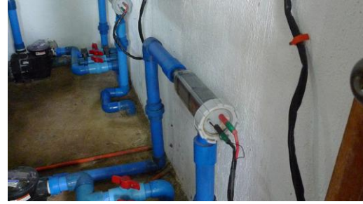
Chlorinator system for the pool utilizes 50 percent less chlorine than traditional methods
