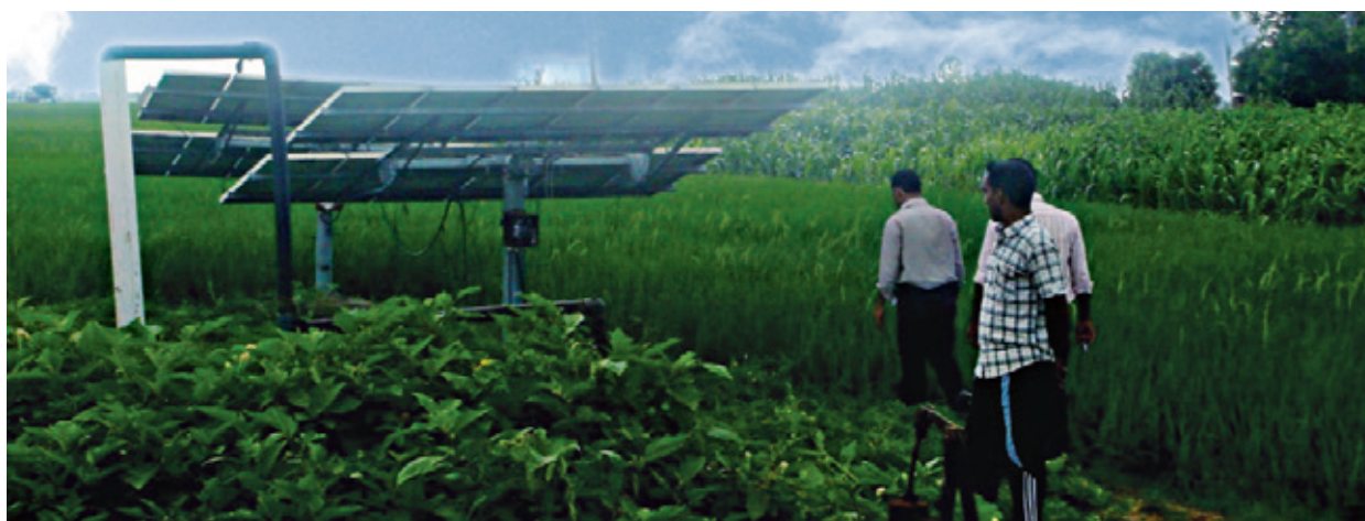
Pump installed under MNRE Solar Water Pumping Programme, Dadri Majra Village, Punjab Picture Courtesy: Thomas Pullenkav
