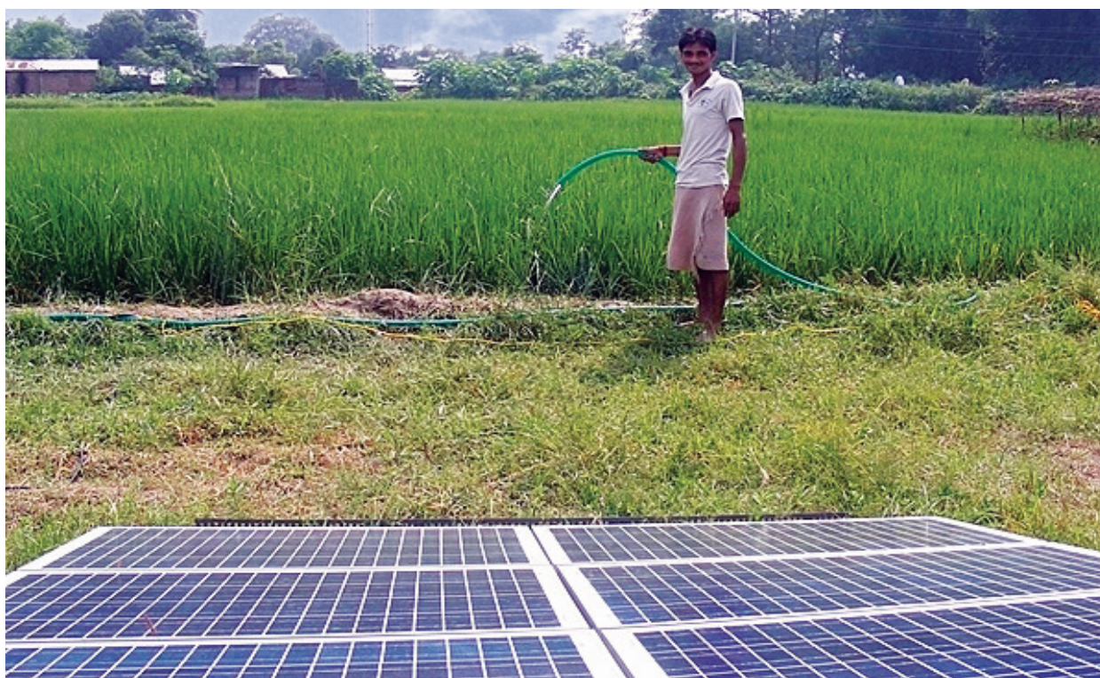
Atom Solar Pump installed in Bihar Picture Courtesy: Greenpeace
