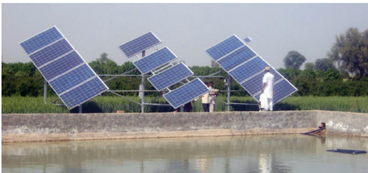
Solar Water Pumps Installed at Nalanda District of Bihar Picture Courtesy: Claro Energy Pvt. Ltd.
