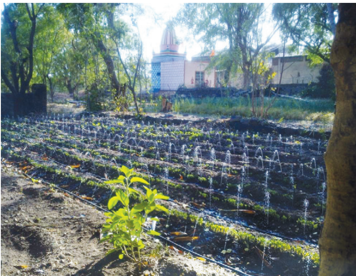
Solar Pump combined with drip irrigation installed near Pune Picture Courtesy: Atom Solar Systems
