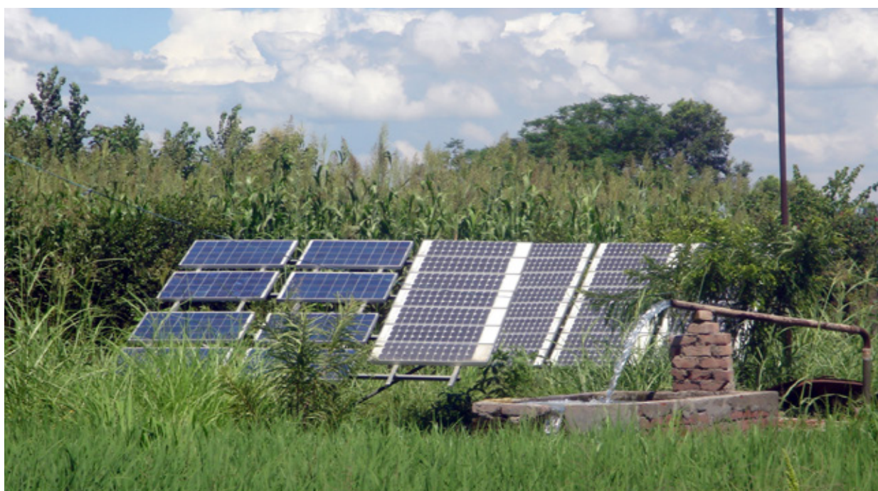
1,800 Wp surface pump in Landra village, Punjab. Picture Courtesy: Thomas Pullenkav
