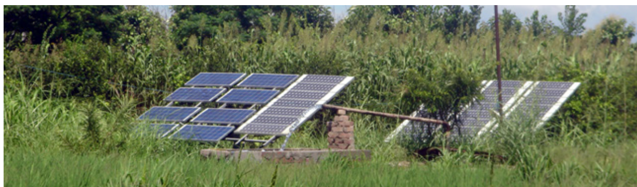
1,800 Wp surface pump in Landra village, Punjab
