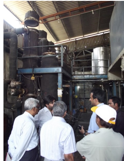
Image no. 21: Installed Caustic Recovery Unit by Textile Industry [Source: GIZ-IGEP and GCPC team]
