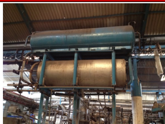
Image no. 25: Hot Water Generation & Storage Tank to Supply Hot Water to Jigger Machines [Source: GIZ-IGEP and GCPC team]
