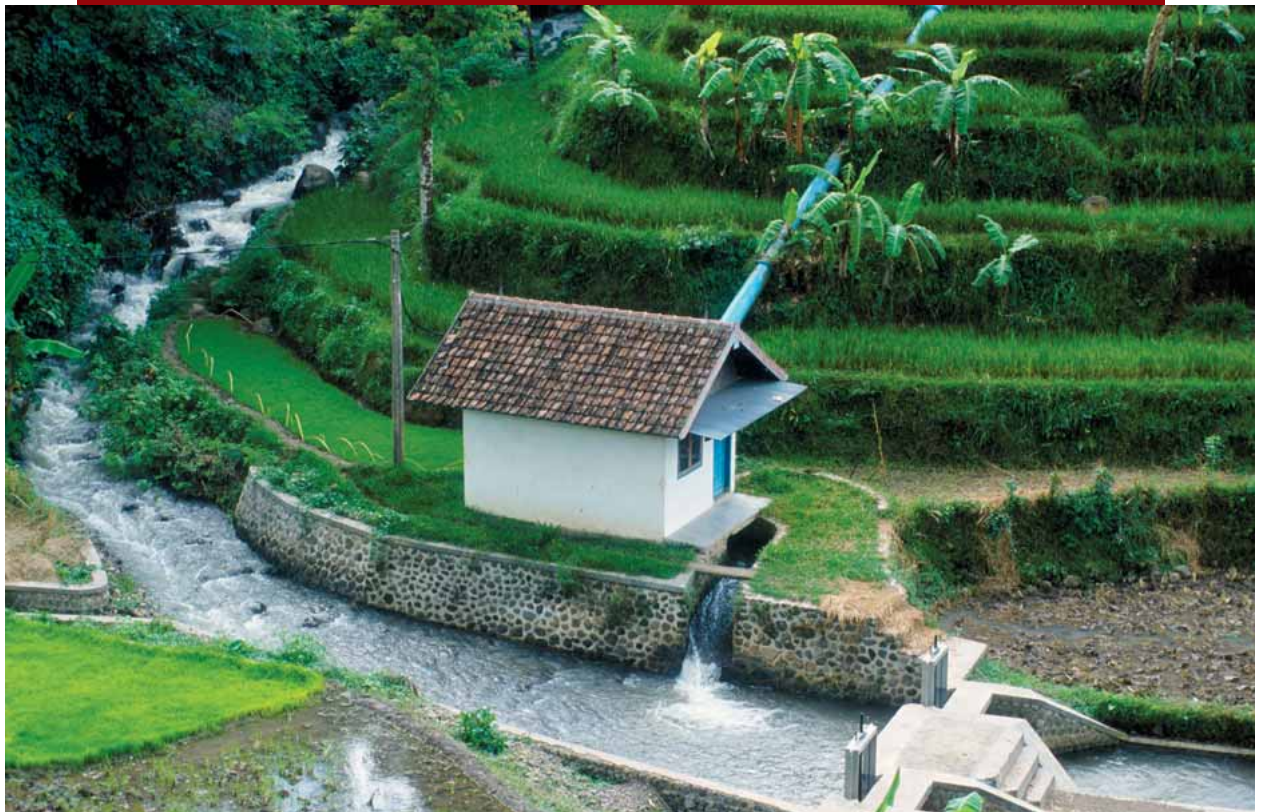
Small hydro-power plants, like in Indonesia, supply rural areas with sustainable energy.
